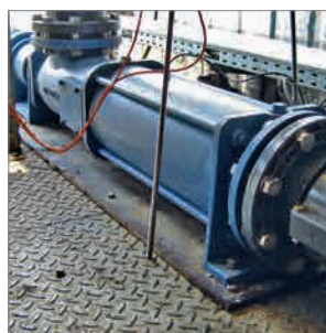
Pumping substrate between fermenters
